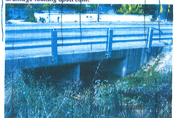
Photo 6. View of the culvert under Sunrise Blvd through which the unnamed drainage exits the Property.
